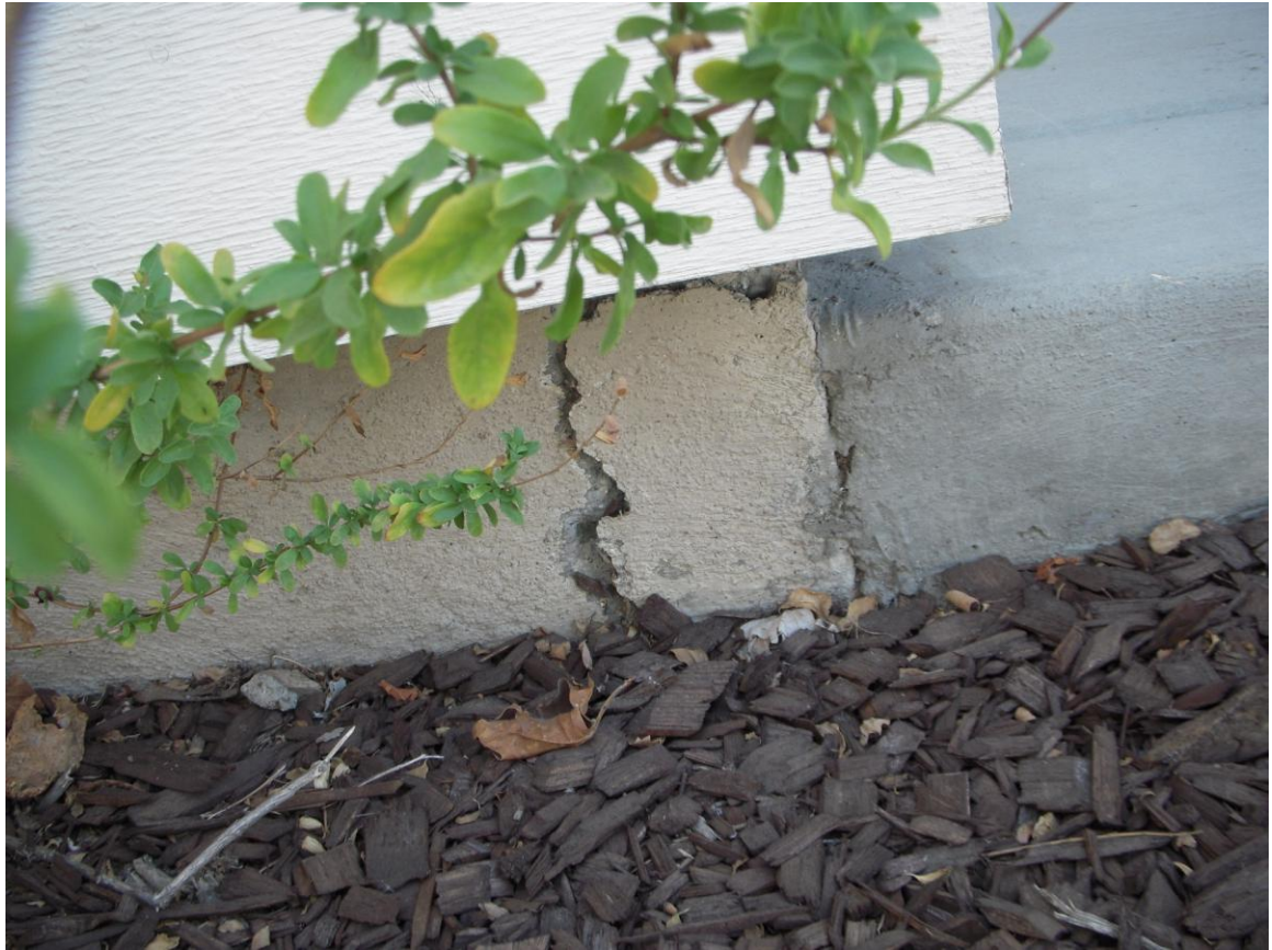
Cracks at the footing, Recommend repair it
